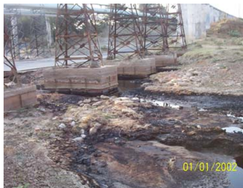
Figure 2.4: Corroded Pillars of Bridge
