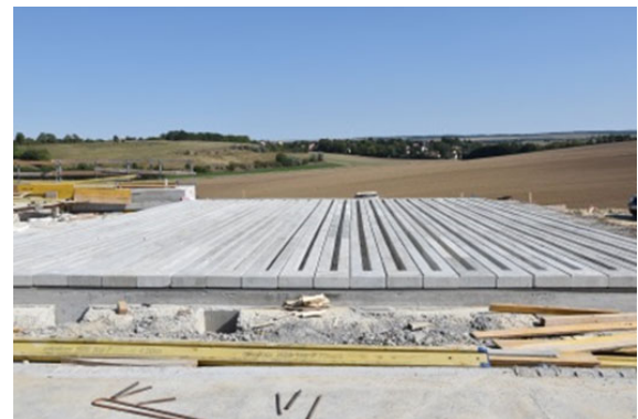
Fig. 1: Construction of the pilot on the Austrian motorway in 2017 by the Austrian motorway operator ASFINAG: A5, Satzengrabenbrücke
