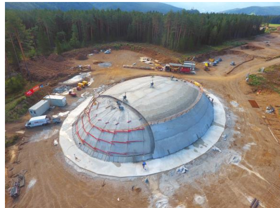
Figure 1: Inflated dome - pilot construction realized in 2017 by ÖBB, the Austrian rail operator as a wildlife crossing over railroad tracks
